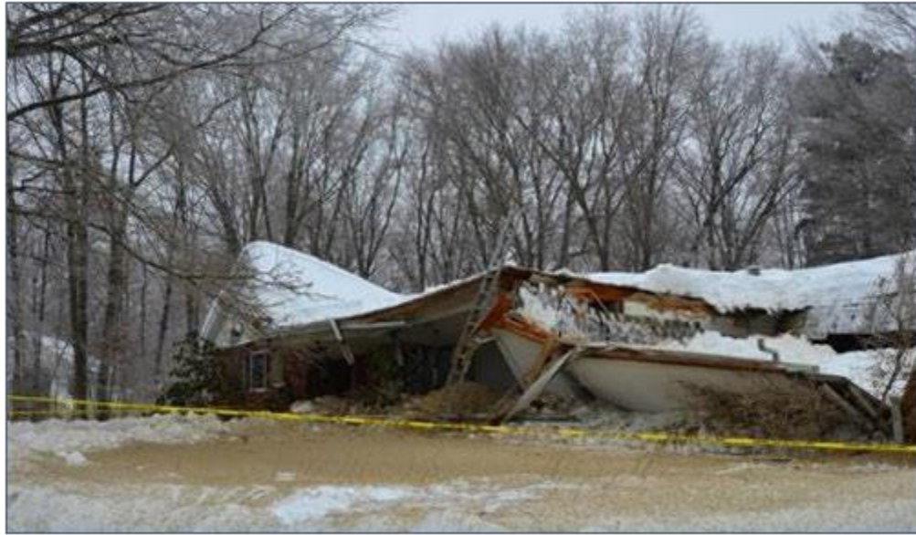
Hebron Building Collapse due to Heavy Snow Loads, February 2, 2011
