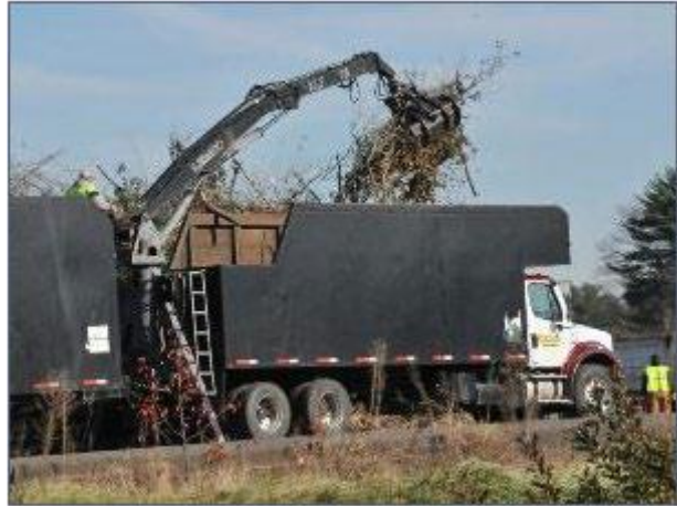
October 2011 Storm Cleanup in Windsor, FEMA
