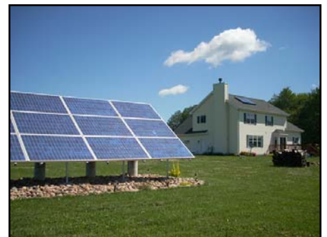
Residential solar array
