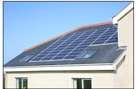
Solar collection system
