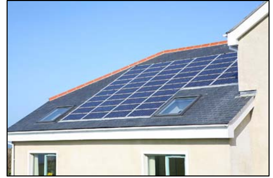
Solar collection system
