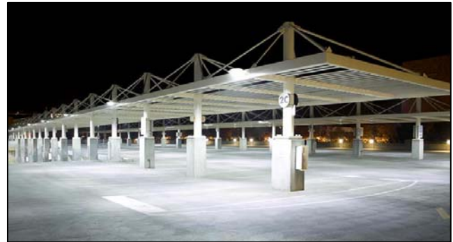
Parking lot lighting
