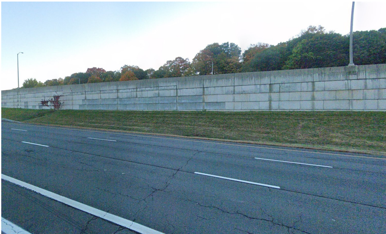
Figure 8 - Retaining wall supporting ramp 84-E-813 with the mainline of I-84 westbound in the foreground
