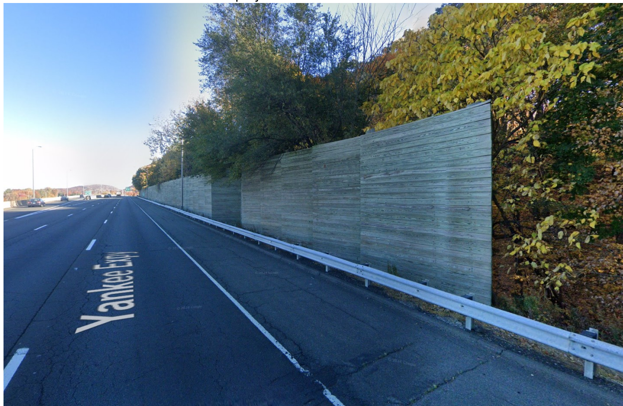
Figure 6 - RB-350 guiderail present in front of the noise barrier wall on I-84 eastbound
