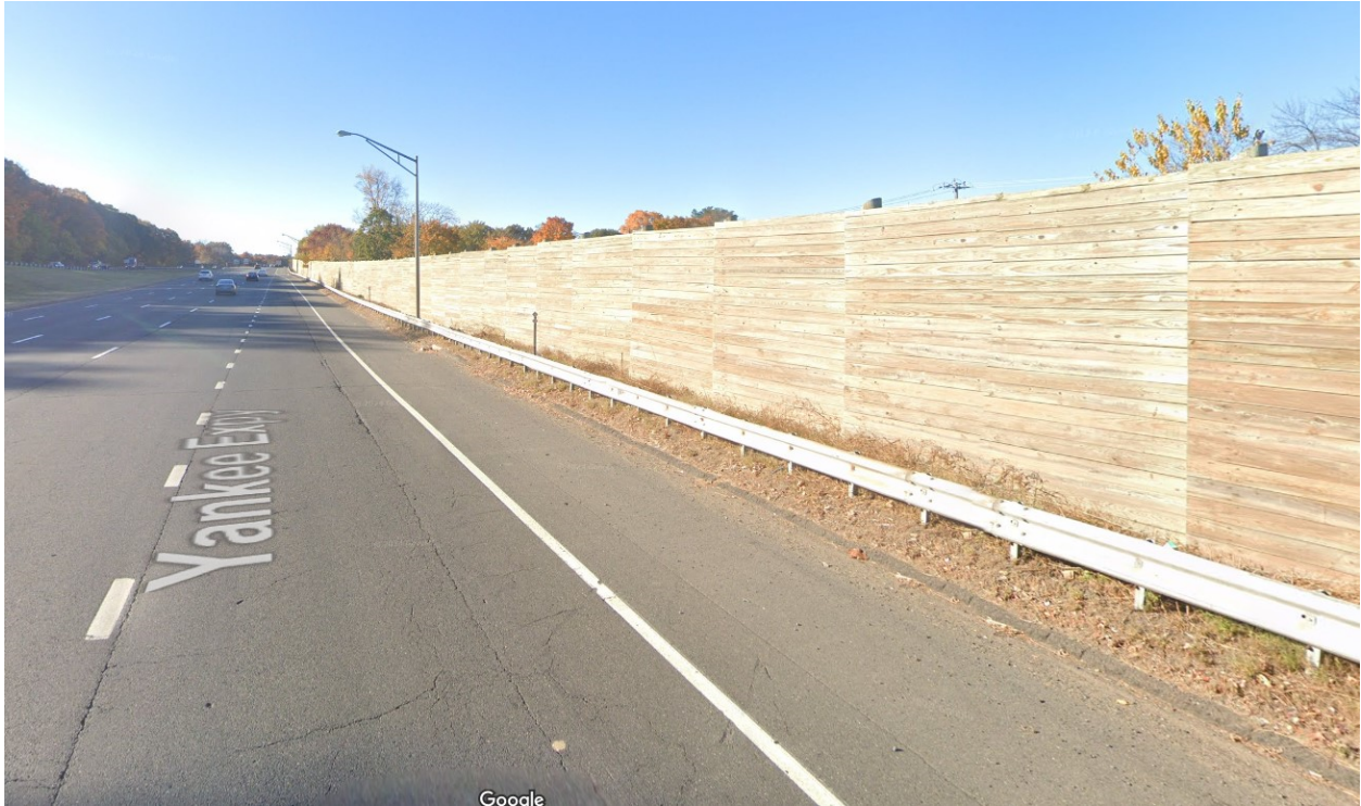
Figure 2 – RB-350 guiderail present in front of the noise barrier wall on I-84 westbound
