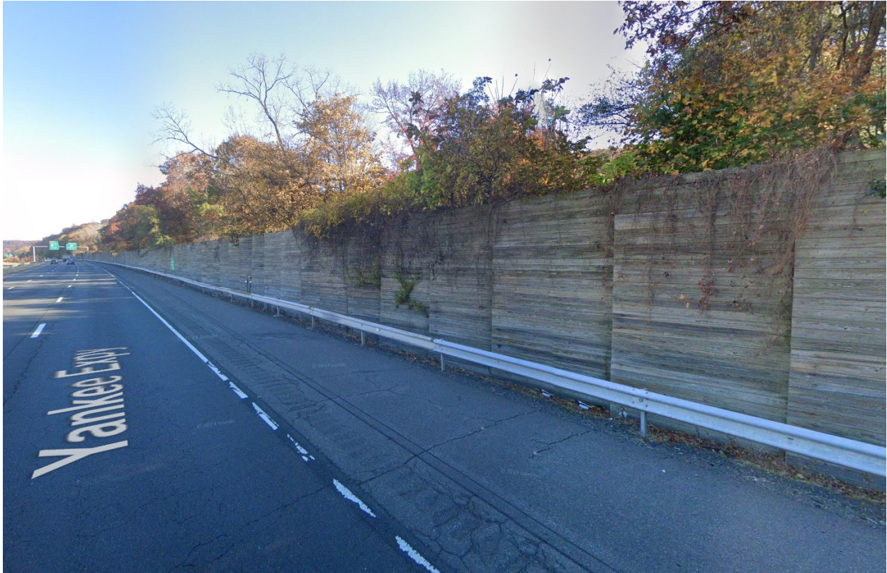
Figure 5 - RB-350 guiderrail present in front of the noise barrier wall on I-84 eastbound
